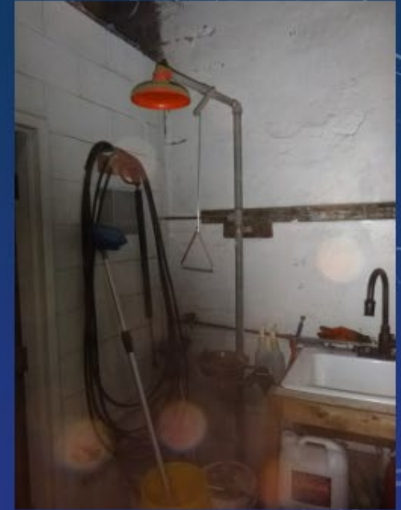
No Hot Water to Eye Wash, No Floor Drain, Outdated Fixtures.
