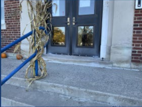
Deteriorated Doors, Non – ADA Entry
