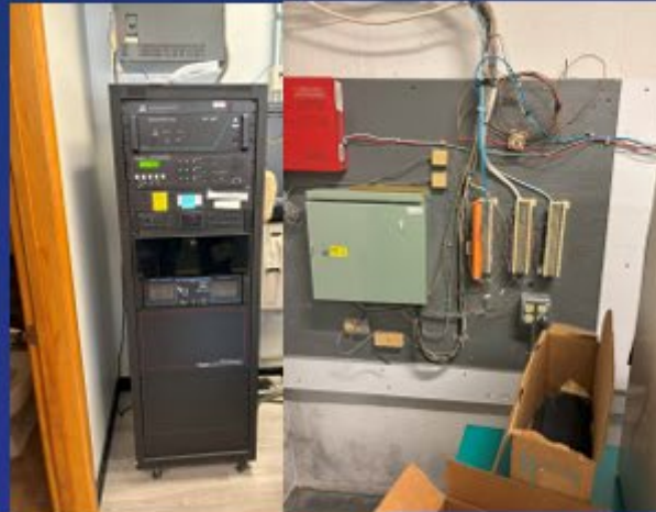
PA System / Clock / Fire Alarm / Mass Notification Upgrades
