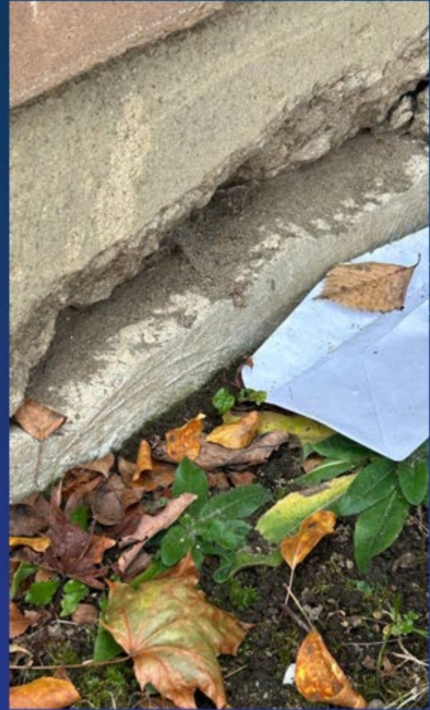
Water Infiltration / Waterproofing
