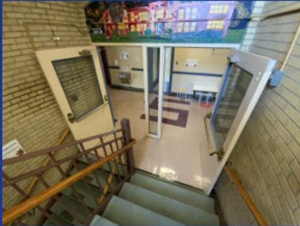
Non-Conforming Accessible Routes
