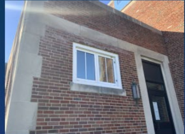
Efflorescence Present, possible moisture
