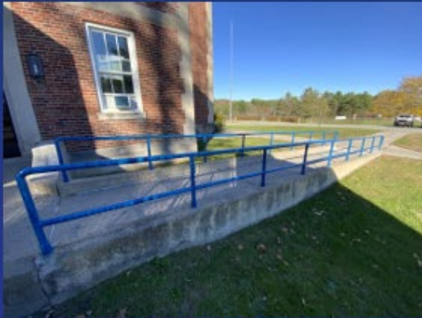
Non-Conforming ADA Ramp / Railing
