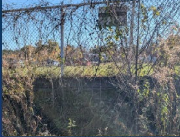
Deteriorated Fencing & Retaining Walls
