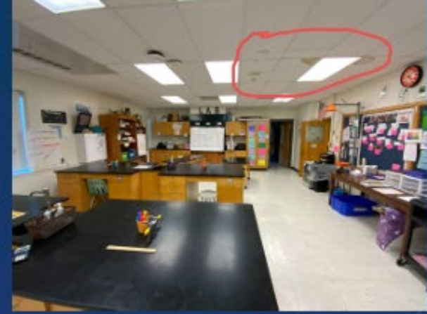
Ceiling Deterioration / Damage Non-Accessible Casework
