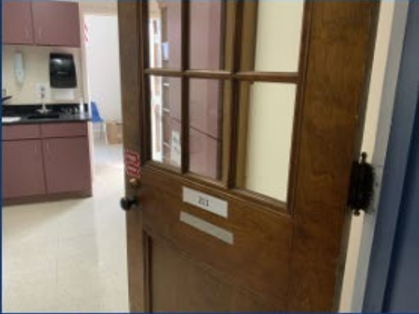
Non-Conforming Doors (Hardware / Rating)
