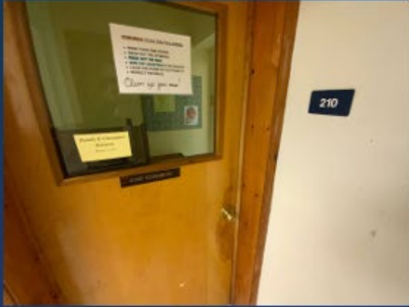
Non-Compliant Doors & Hardware
