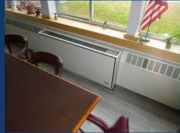
Unit Ventilator / PTAC Replacement / Relief Air
