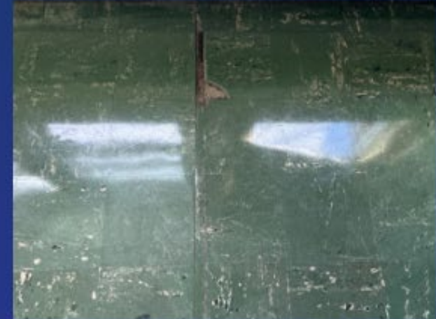
Flooring / Structural Cracking
